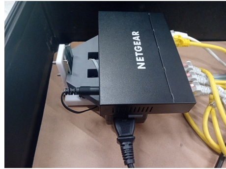
Figure 6: Ethernet hub mounted on the new support piece, now fitting the box
